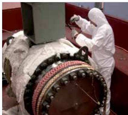
High temperature valve testing
