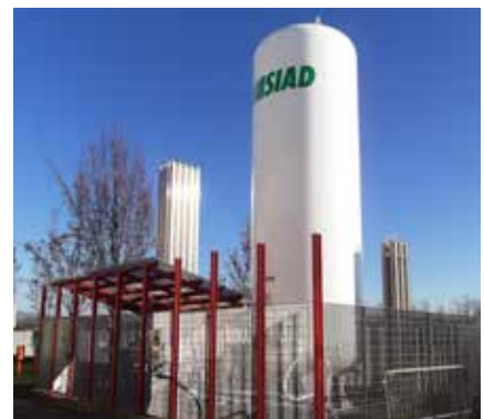
High Pressure System for Gas Testing
